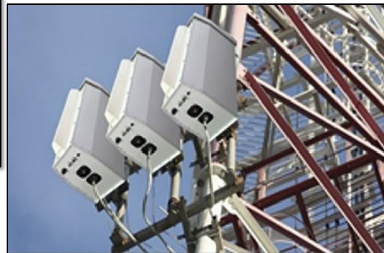
Pole-21 stationary unit attached to cell tower. Source: © 28 March 2023, Focus.ua 127
